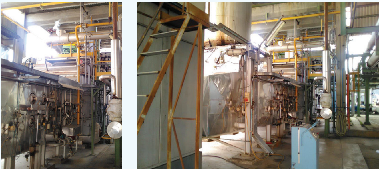
Figure 1 Exhaust gases vent and recovery boiler - Co-Generation System - Campoverde di Aprilia Plant
