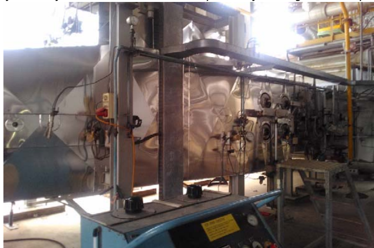
Figure 1 - Channelling of emitted fumes into the steam recovery boiler of the co-generation system
